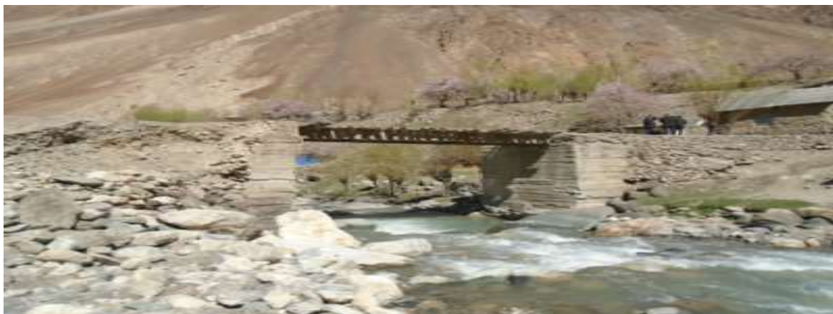
Photo: Current condition of Bridge No.2 in Yazgulom jamoat of Vanj district
